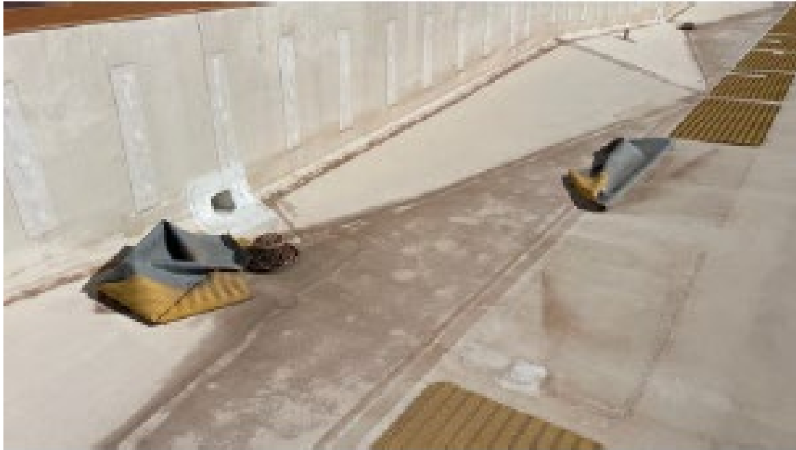
Damaged walk pads
