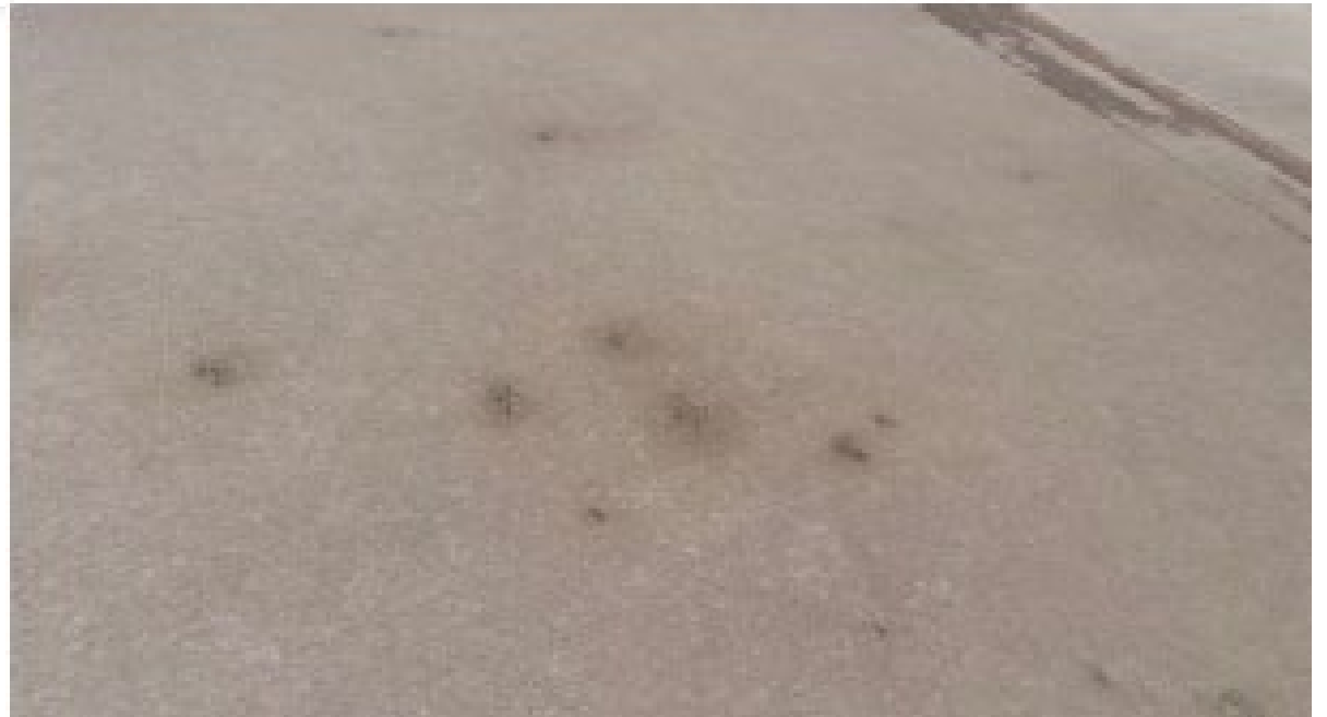
Observed hail Damage
